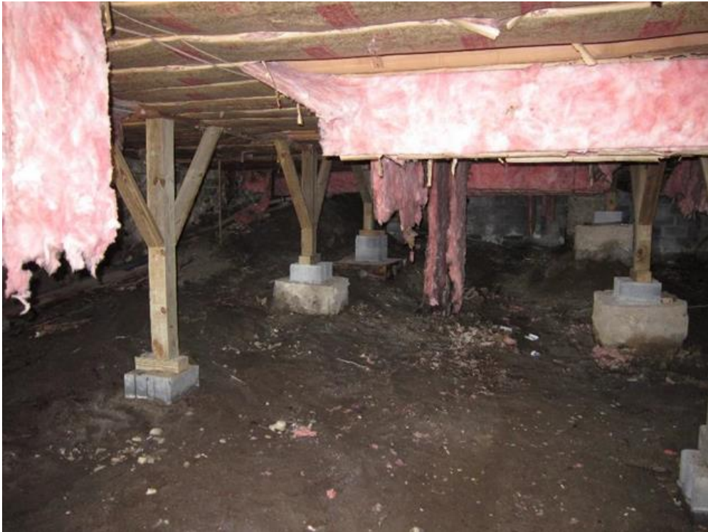
From dark and damp (above) to a finished lower level (right, shown in progress)
